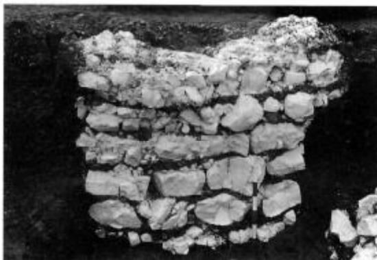
Fig 16. Section through the foundation of phase 2 church on the south side, looking east (for position see Fig 6). Scale is 5 × 100mm units
